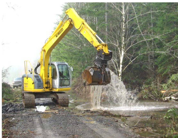
Beavers cause damage to culverts, potentially causing damage to roadways and forcing increased maintenance and repairs by landowners.
