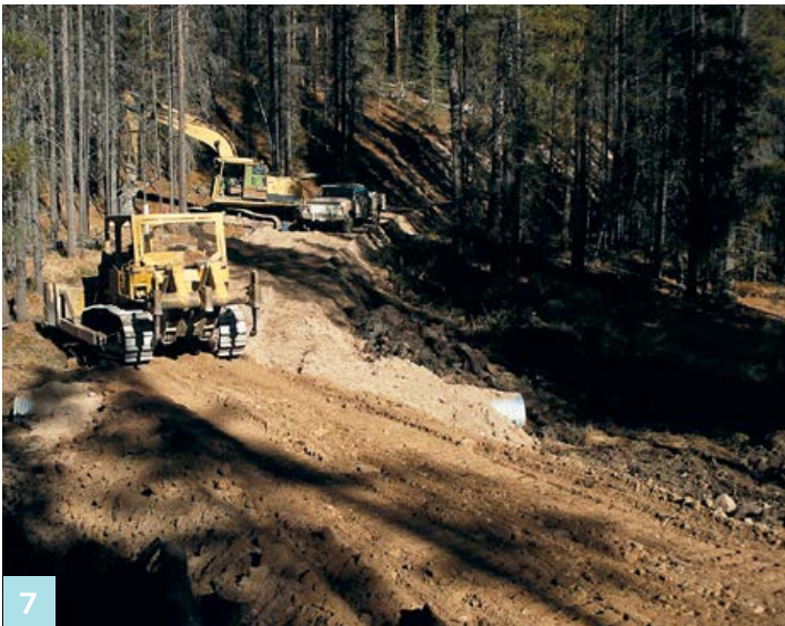
7 Layers of fill are pushed into place and carefully compacted to build up and maintain a consistent road grade. The crossing should be rocked to minimize the risk of sediment washing off the road and into the stream.
