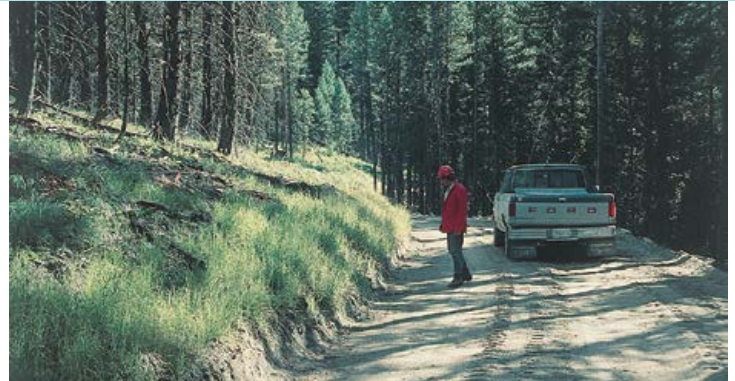
Grader damage to inside ditch toe slopes exposes an easily erodible surface and is a source of sediment.
