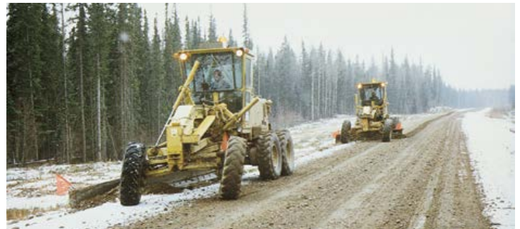
Slow, controlled grader operation is key to reducing culvert inlet and outlet damage. Reduce damage by keeping graders on the road running surface. Never sidecast gravel toward culvert inlets or outlets.
