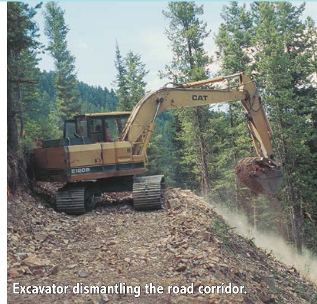
Road segment before vacating.
