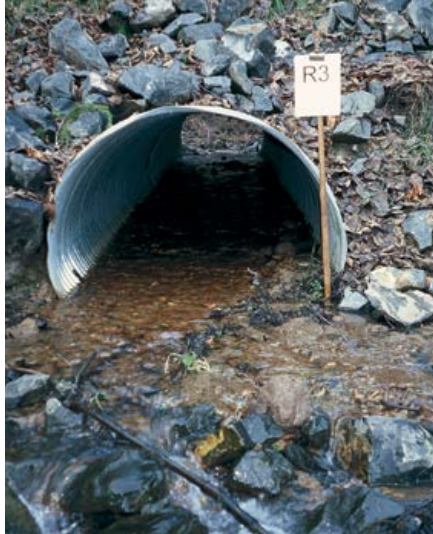
Round, galvanized corrugated metal pipe sunk into the streambed to allow for fish passage.
