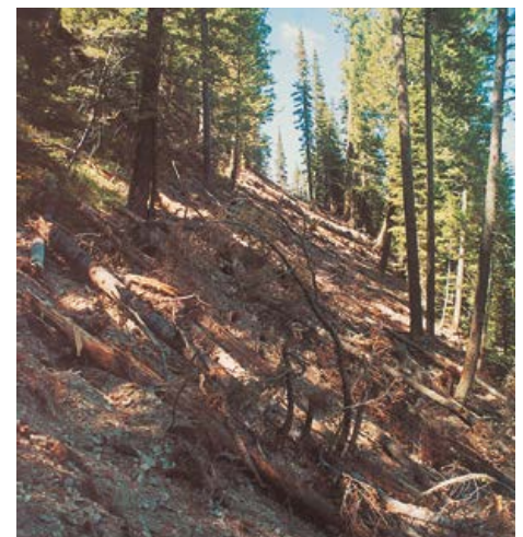
Vacated road segment with large wood in place before reseeding the surface with grass.
