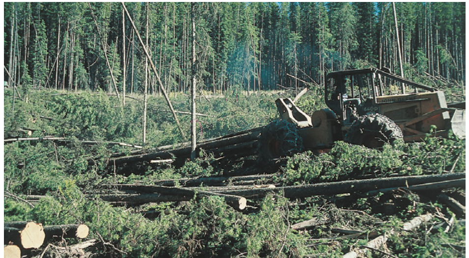
Skidders or dozers drag logs from the forest to the log landing. To reduce soil disturbance, rubber-tired skidders or crawler tractors should be kept on skid trails. Winch line and chokers pull logs to the machine.
